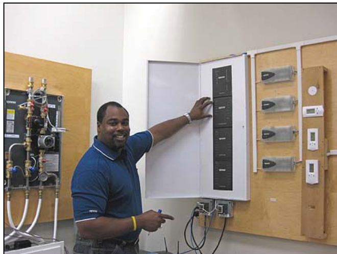
Senior Trainer Wes Sisco instructs students on essential design fundamentals and offers hands-on training for installation and troubleshooting techniques.
