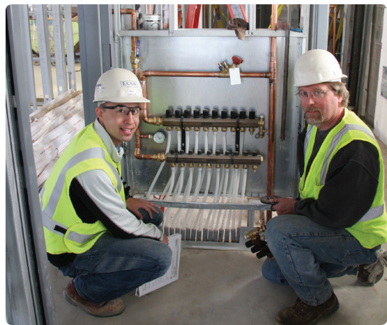
Figure 4-3: Manifold in Flush-mounted Wall Cabinet (See Uponor Product Catalog for available sizes.)
